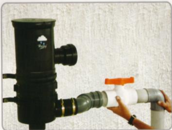
2. Fix 75 M.M. Control Valve (First rain flush out valve), with suitable elbows and fixtures.
