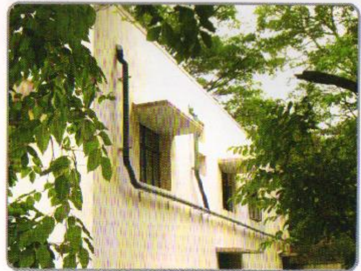
2. Inter connect the down flow pipes and draw the line till the point of Filter location
