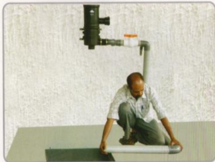
3. Connect the delivery line to the sump with necessary length of Pipeline with Fixtures.
